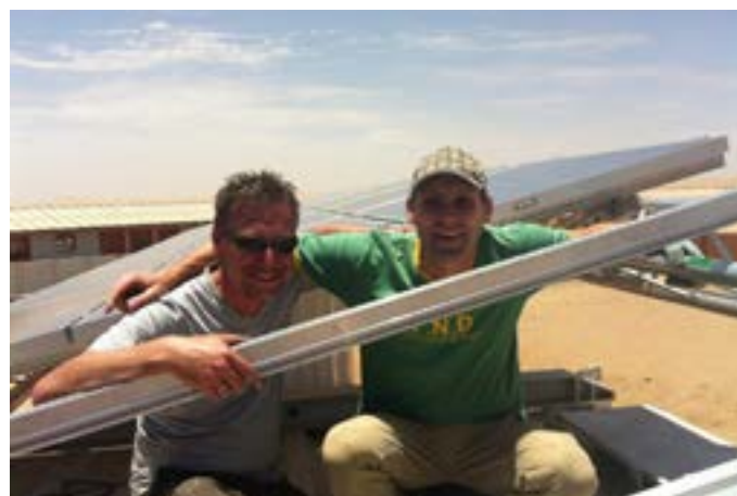
Figure 6.2 YA Namibia - Dirk Bellens and Dick Neuteboom assembling the mobile solar energy station
