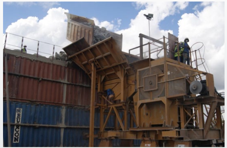
Crusher plant at Namialo Quarry (10th July of 2012)
