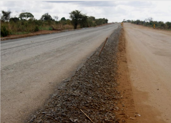
1st layer of crushed stone base already done 'left hand side' (10th July of 2012)
