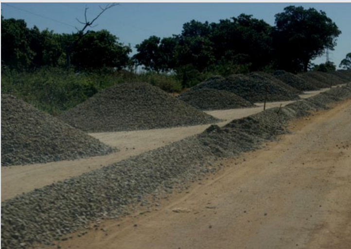
1st layer of crushed stone base completed with material for 2nd layer already on site (13th July of 2012)
